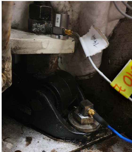
Figure 21: SBN sensors at engine mounting of 4EW, attached with magnet above resilient mount, attached with plate and adhesive below resilient mount
