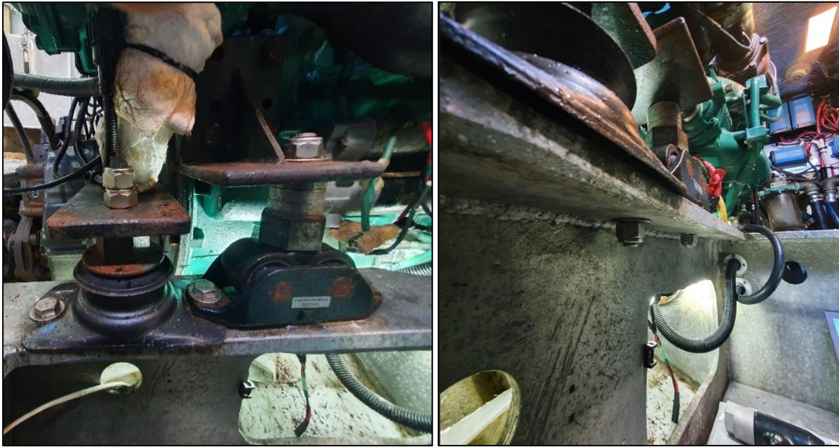
Figure 73: engine foundation on GW
