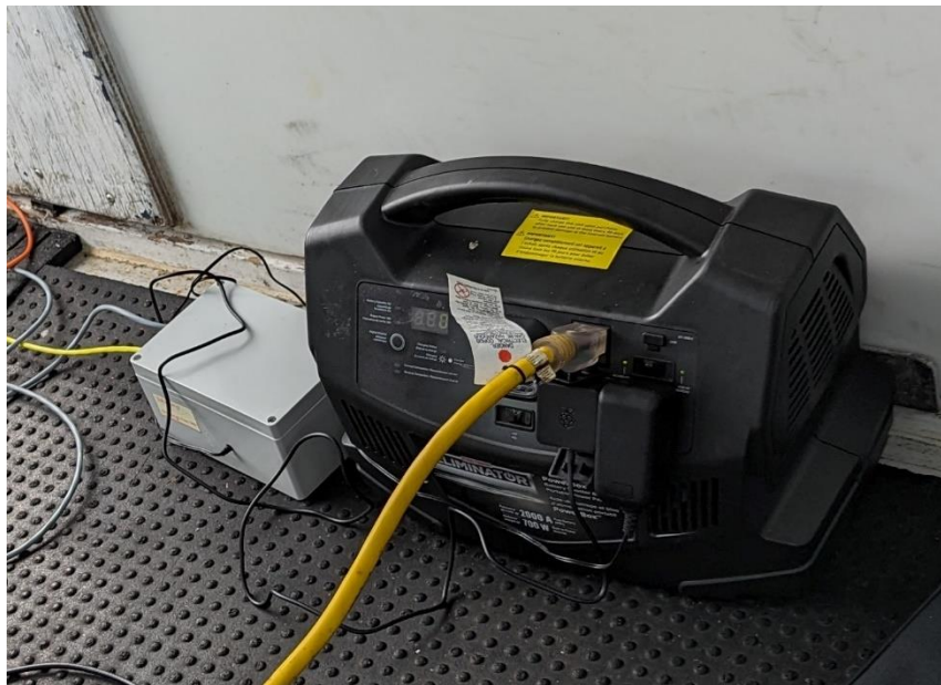
Figure 5-3 CBM system in-situ on a fishing boat trial powered from a portable power pack.
