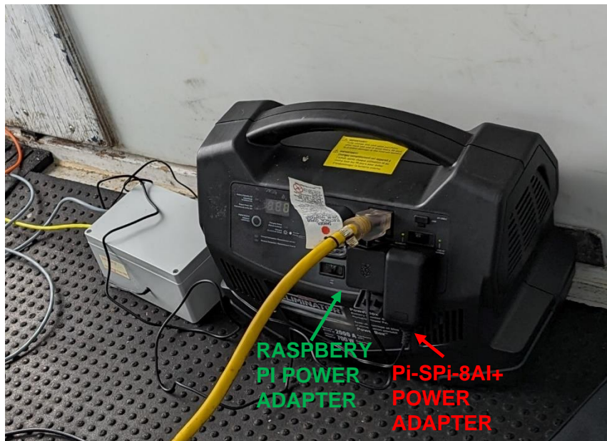
Figure 3-2 CBM system in-situ on a fishing boat trial powered from a portable power pack.
