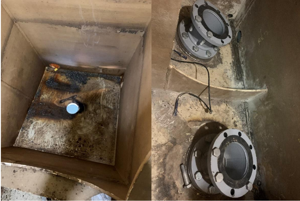
Figure 4. Installation of the sensors used to measure cavitation. (Left) Hole drilled through hull, and (right) pressure glands being installed around the sensors. Photos by Mount Royal Walsh installation team.
