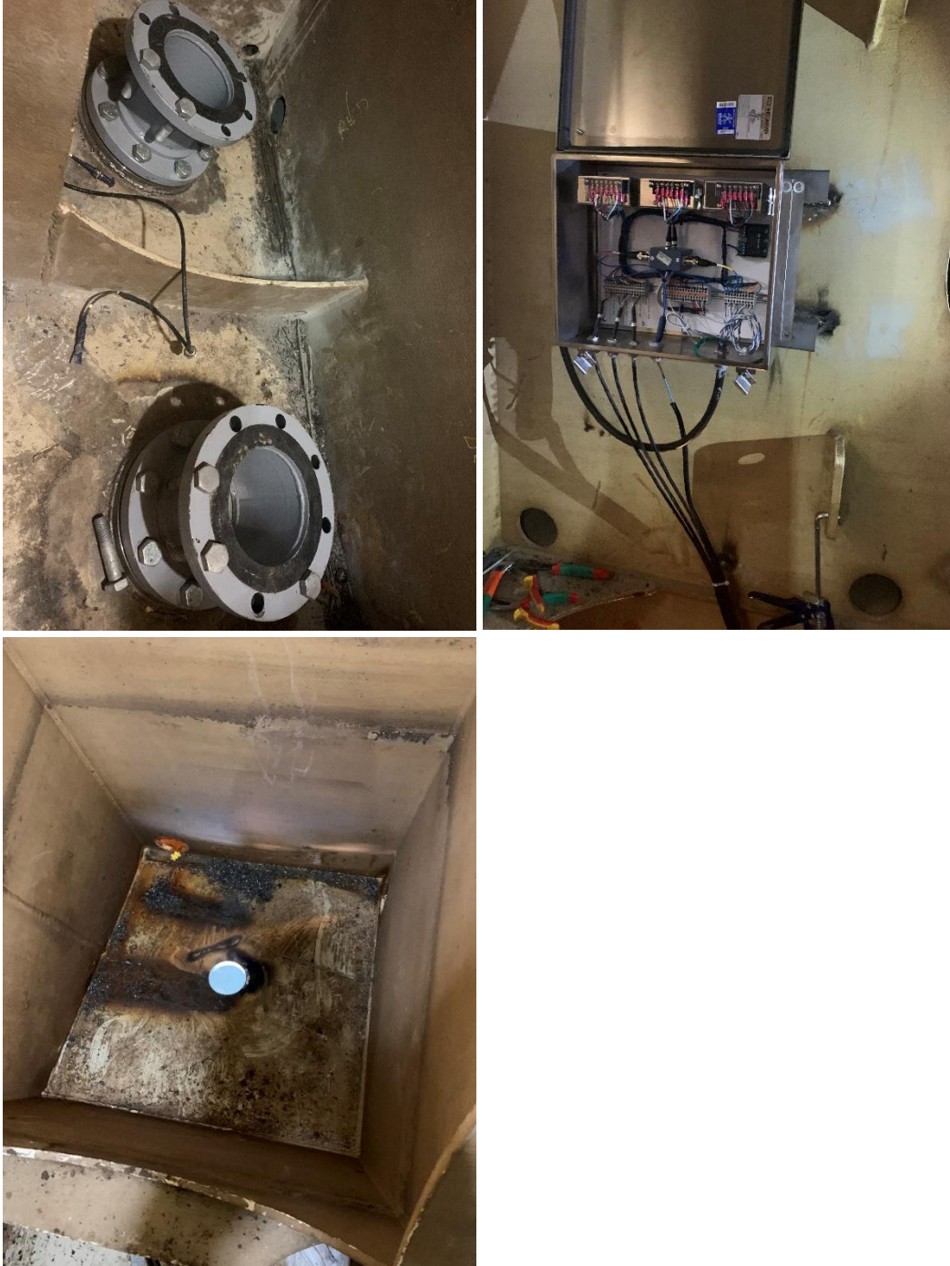
Figure 11. Location and installation of the sensors used to measure cavitation. Photos by Mount Royal Walsh installation team.
