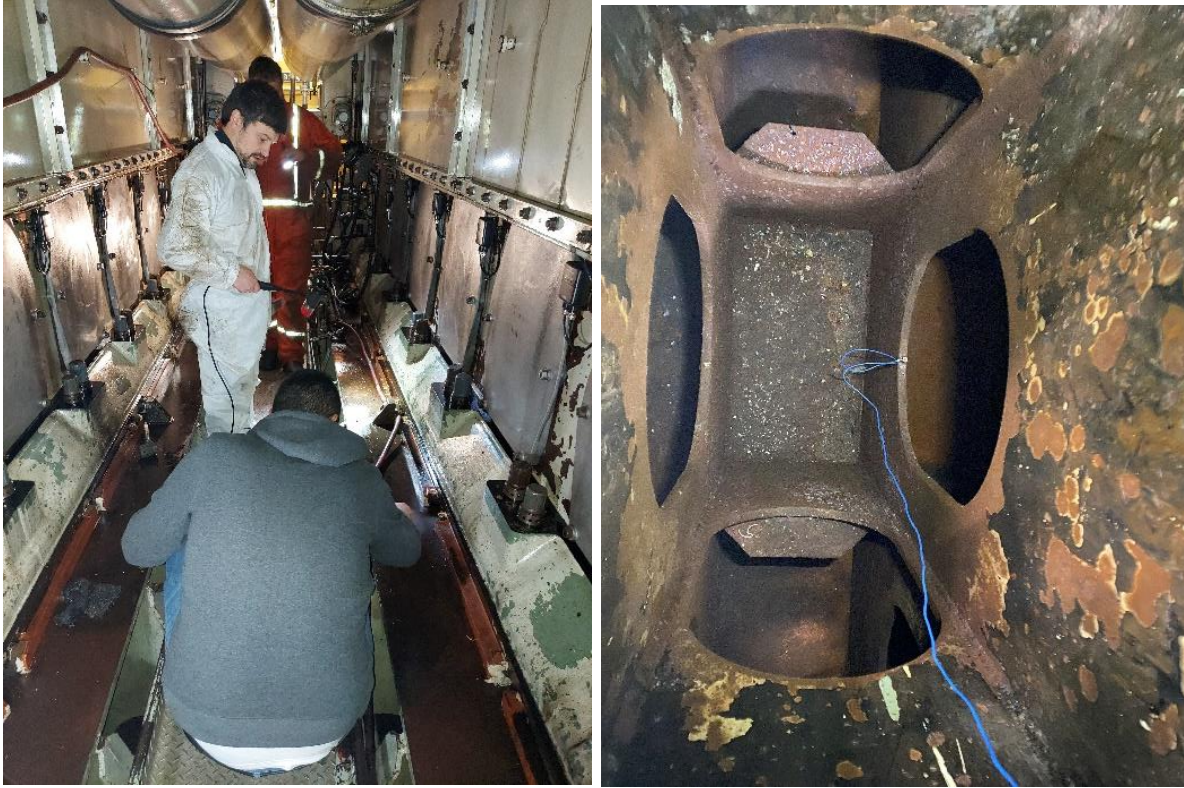
Figure 2-9 Accelerometer installed in the ship double bottom and at machinery base
