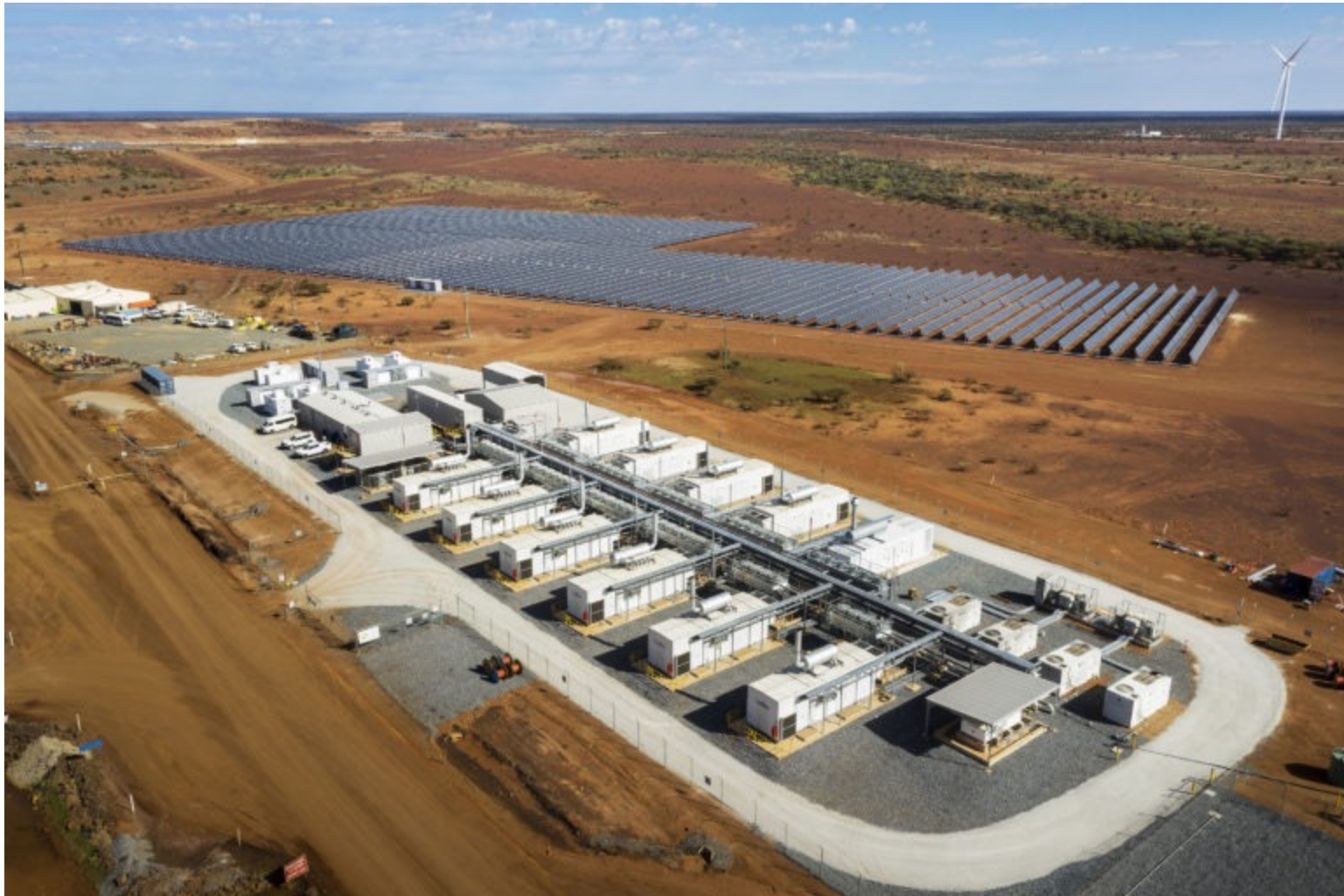
Gold Fields' Agnew gold mine in Western Australia. The 56-megawatt (MW) Agnew hybrid renewable microgrid system
